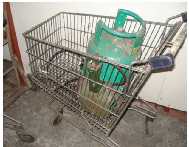
Unsafe storage of gas cylinders
